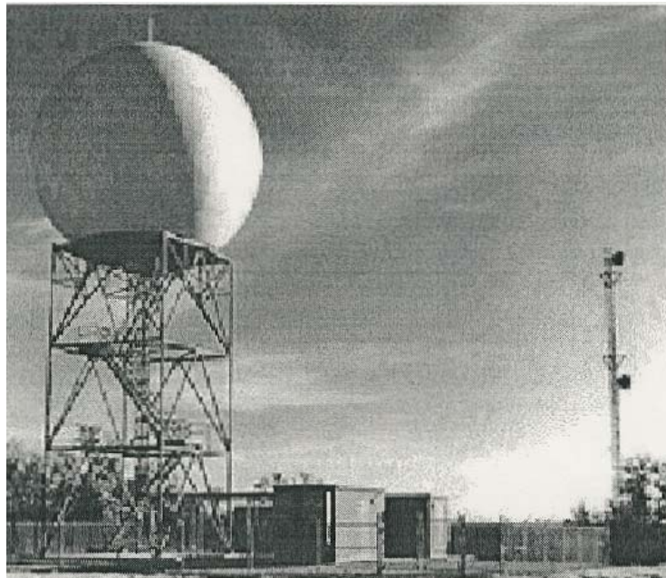
Figure 1-2 NEXRAD Radar Data Acquisition (RDA) unit.
